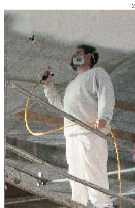
Putzmeister airless devices can be used for an amazing range of applications. Here, for example, a hall ceiling is being sprayed with paint.
