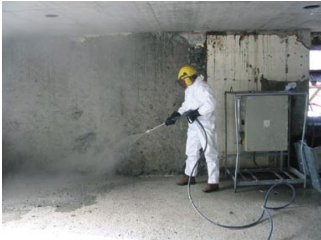
With 500 bar water pressure, the old plaster was easily removed – quickly, cleanly and free of dust.
