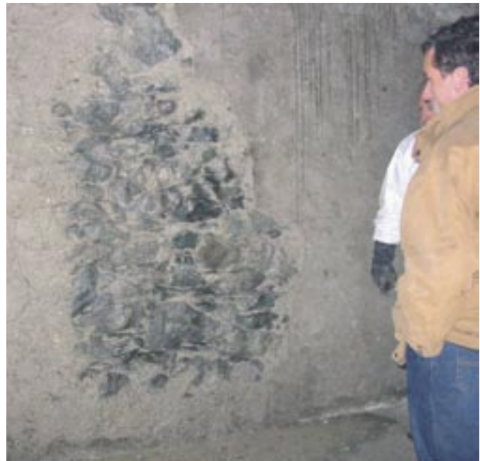
Here you can see a part of the original granite masonry – after the mortar has been 'tackled' by a 500 bar water jet.
